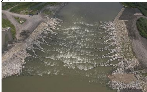
Drone photograph of the nearly complete Drayton Dam project (August 29, 2023). Image courtesy of the North Dakota Game and Fish Department.
