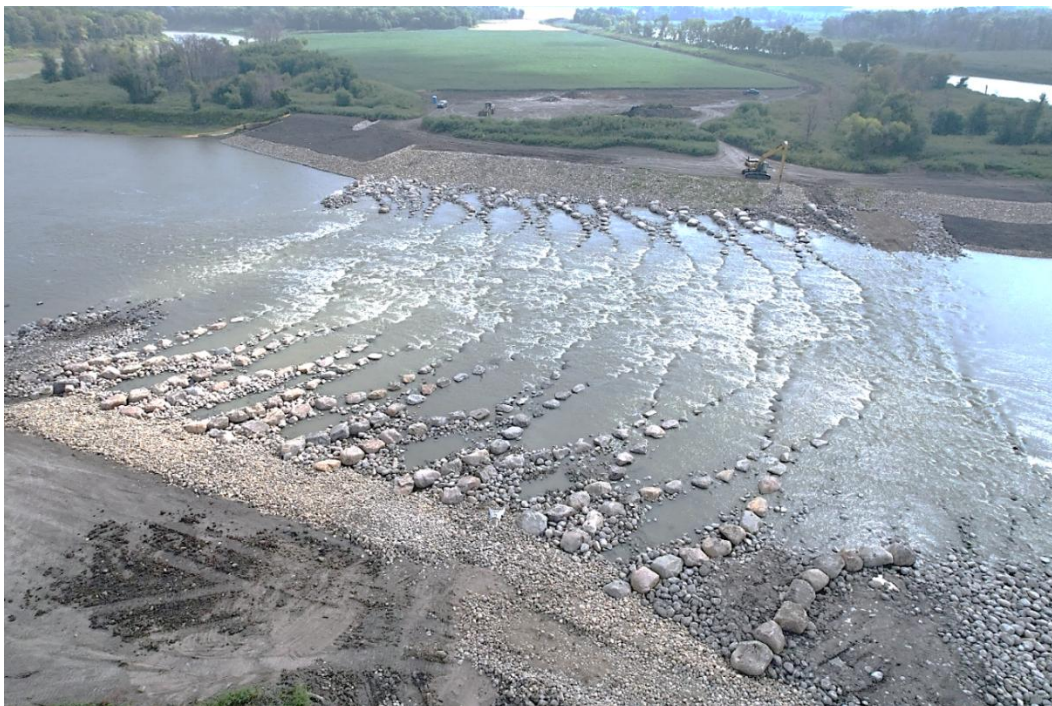
Figure 8: The newly constructed rock-arch-rapids at the former Drayton Dam site, North Dakota.
