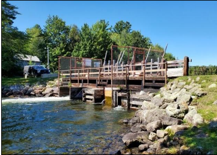
Figure 4 The Forest City Dam located at the outlet of East Grand Lake along the international boundary.
