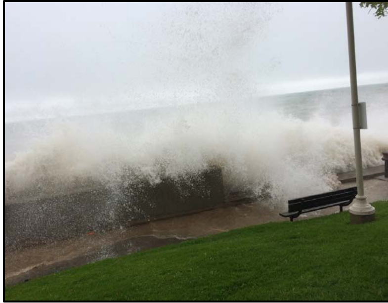
Figure 5-36: Overtopping of shore protection, Stoney Creek, ON. Photo credit: ECCC, May 2017.
